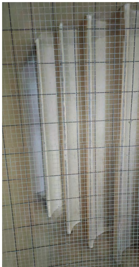
Figure 3.4 Further details of the the turning vanes and 13 mm square mesh safety screen of the DII wind tunnel.
