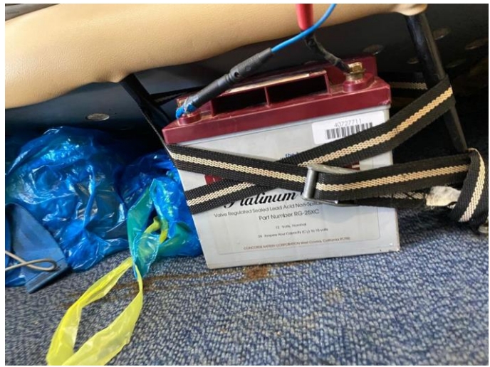
Figure 3.9 ballast and battery
