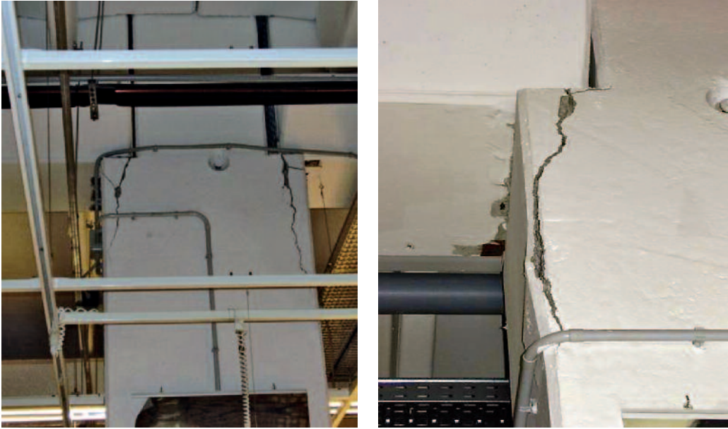
Fig. 5 Local failure of the beam support.
