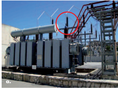
Fig. 5 (a) Damage to rigid connection of a transformer. (b) Typical damage to pedestal box.
