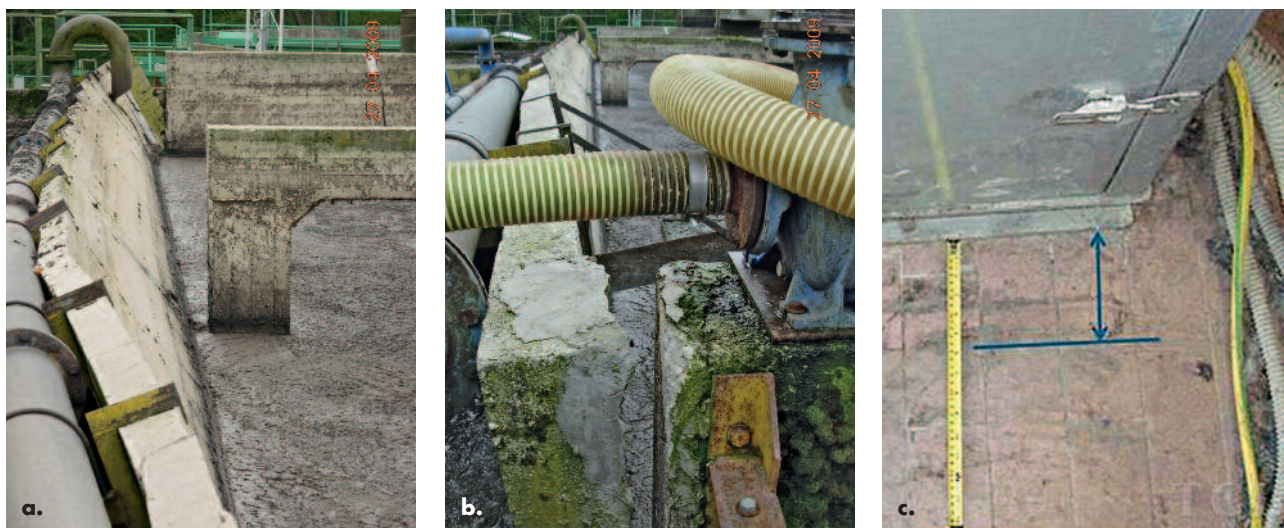
Fig. 3 Ponte Rosarolo Plant. Digestion Tank: (a) partial collapse of a longitudinal wall and of the pipe connected to it. (b) Detail of the detachment of the orthogonal walls at the edges. (c) Displacement of the pump in the control room.
