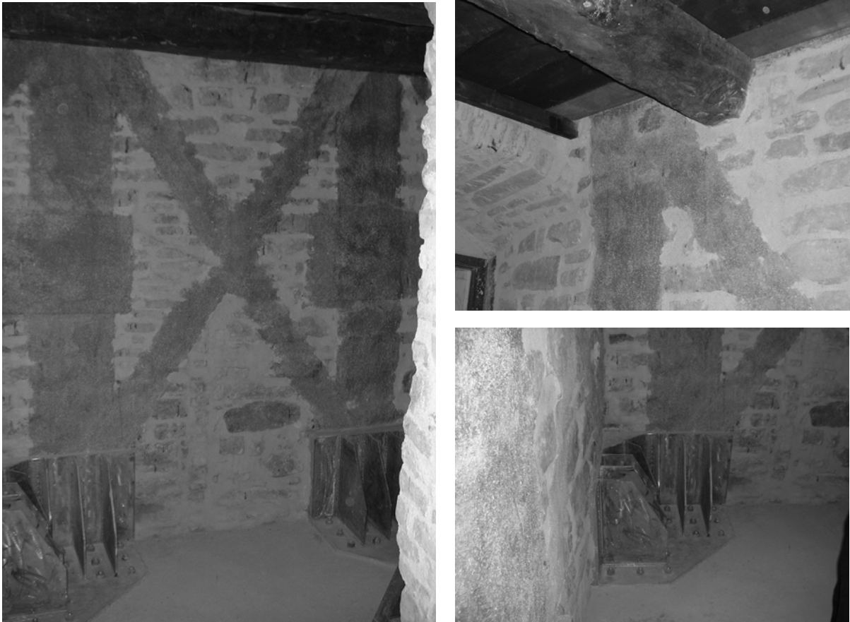
Figure 3. Installed composites and base anchorage. Composites near to un-removed wooden floor. Intervention anchoring details.
