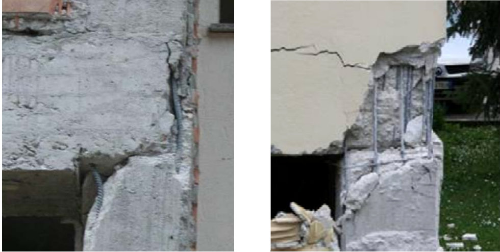
Figure 7.15. Failure mechanisms at joint – column interface surfaces
