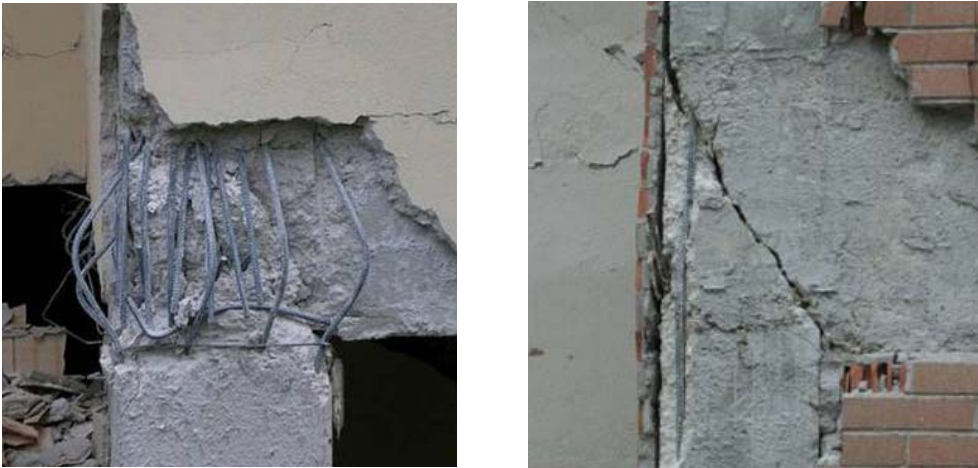
Figure 7.14. Joint failure with evident (a) longitudinal bar buckling and (b) diagonal cracking failure in concrete joint panel.
