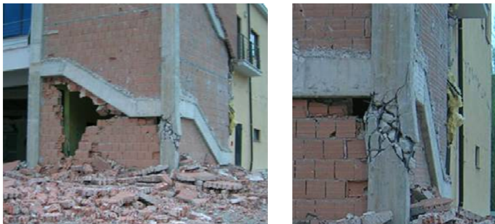
Figure 7.12. Shear failure in squat columns of the staircase.
