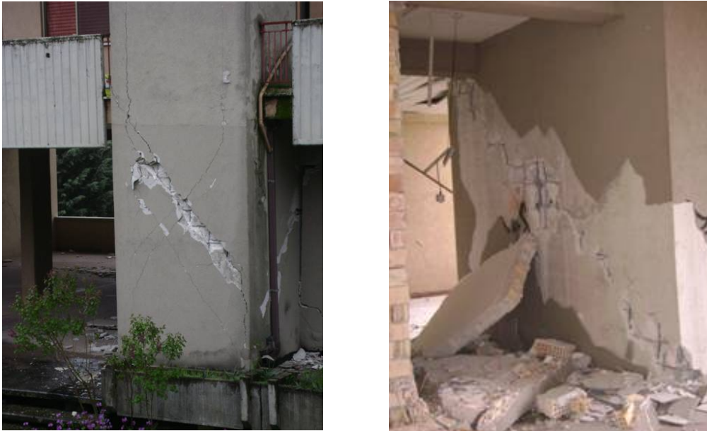
Figure 7.13. Failure in reinforced concrete walls.
