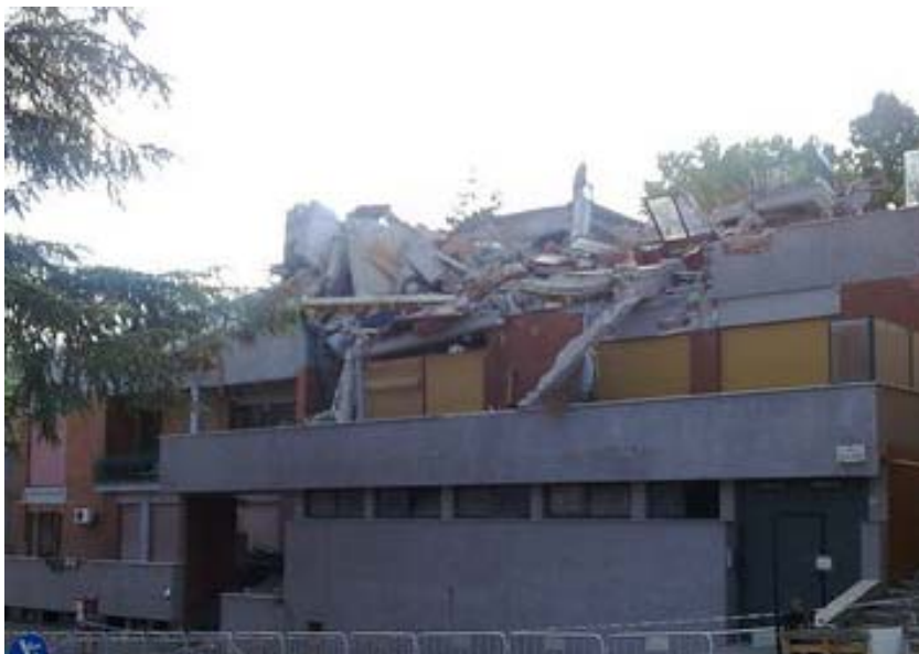
Figure 7.18. Soft storey mechanism examples in L'Aquila: Via Porta Napoli.
