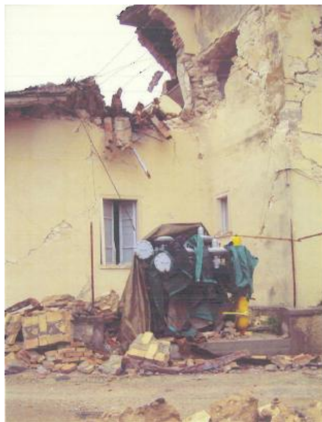
Figure 3. GR housed in a masonry kiosk closed to building and damaged following the 6 th April 2009 earthquake.
