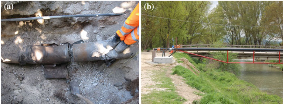
Fig. 6 Damage to gas pipes following the L’Aquila earthquake: a gas welded joint of a LP steel pipe pulled apart in Paganica (AQ); b gas pipe connected to a damaged bridge in Onna (AQ) replaced with a stand-alone pipe (photos courtesy of ENEL Rete Gas)
