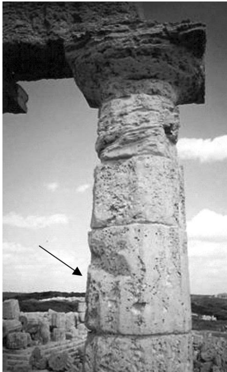
Fig. 2. View of southern elevation of column #7 and the drum chosen for the application.
