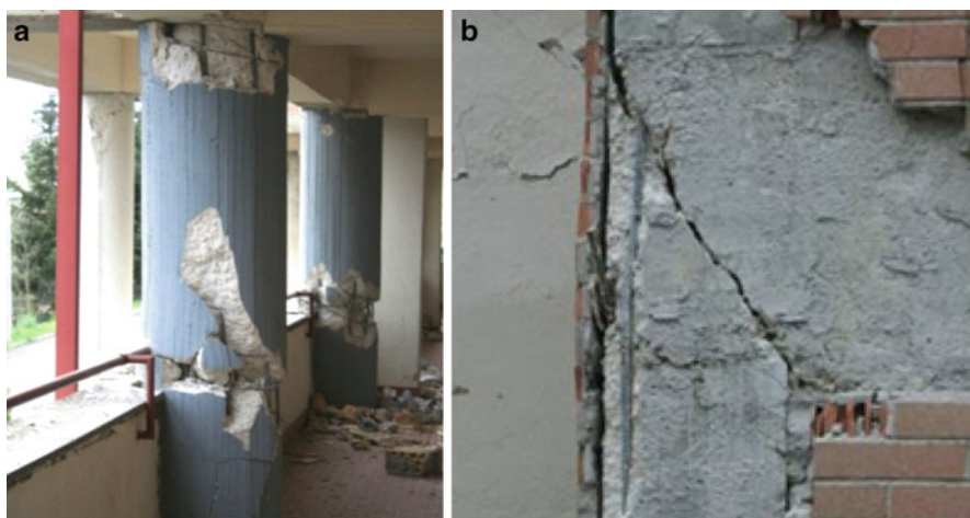
Fig. 10.6 (a) Shear failure of column adjacent to partial infilling panels; (b) diagonal cracking failure in concrete joint panel (Ricci et al. 2011a)
