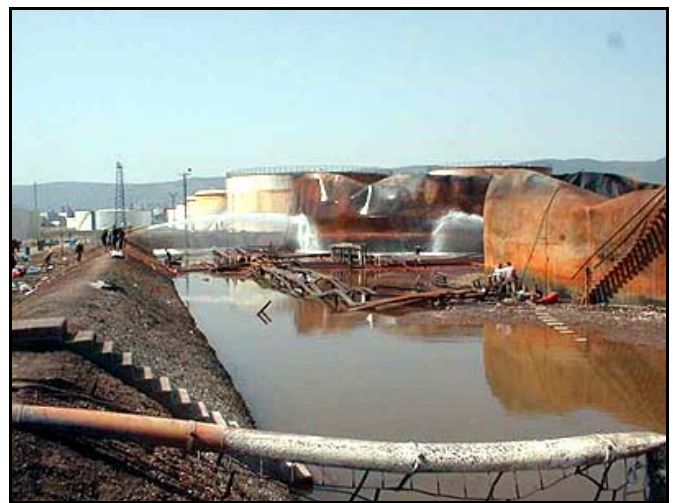
Fig. 1. Tupras refinery (Turkey) after 1999 Koaceli Earthquake. The refinery suffered over $100 million damages [36].
