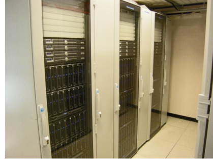
(a) Three rack servers of the data center.
