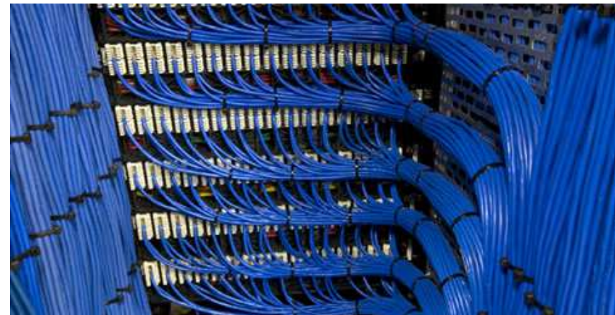
Patch panel for UTP cables: rear view
